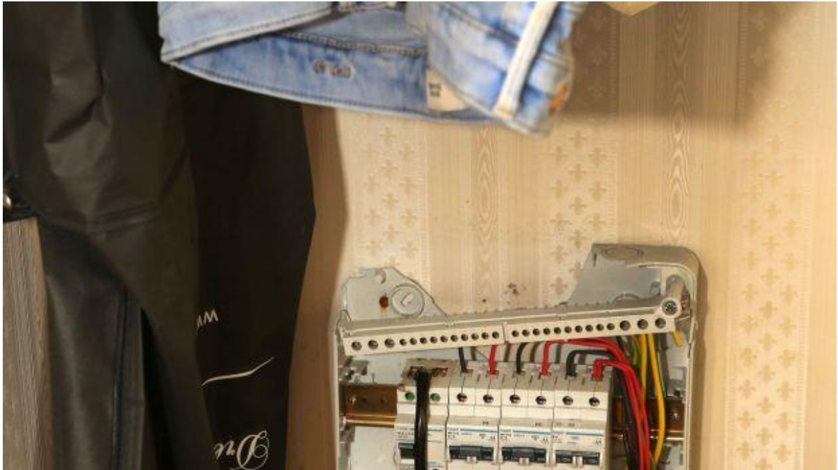
Wiring in a caravan at the Carrowbrowne temporary halting site in Galway. Photograph: Joe O'Shughnessy
